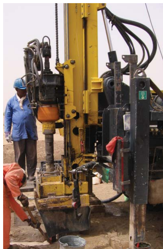
A World Vision drill rig bores a well in the village of Nongon Gochi.
